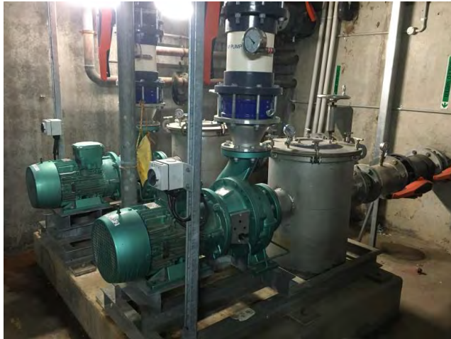
Typical commercial pool filtration pumps.
