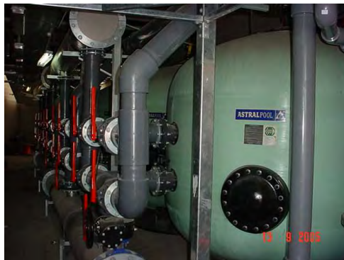
Large commercial sand filters.
