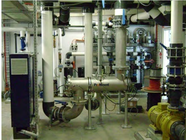
Typical medium pressure UV unit.
