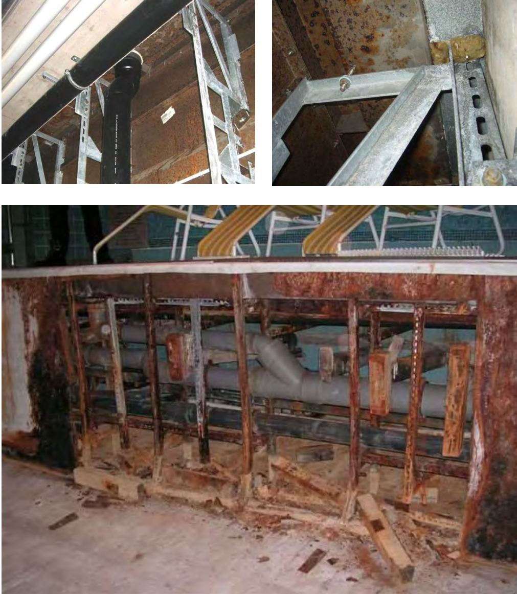
Examples of Corrosion and Panel Failure.
