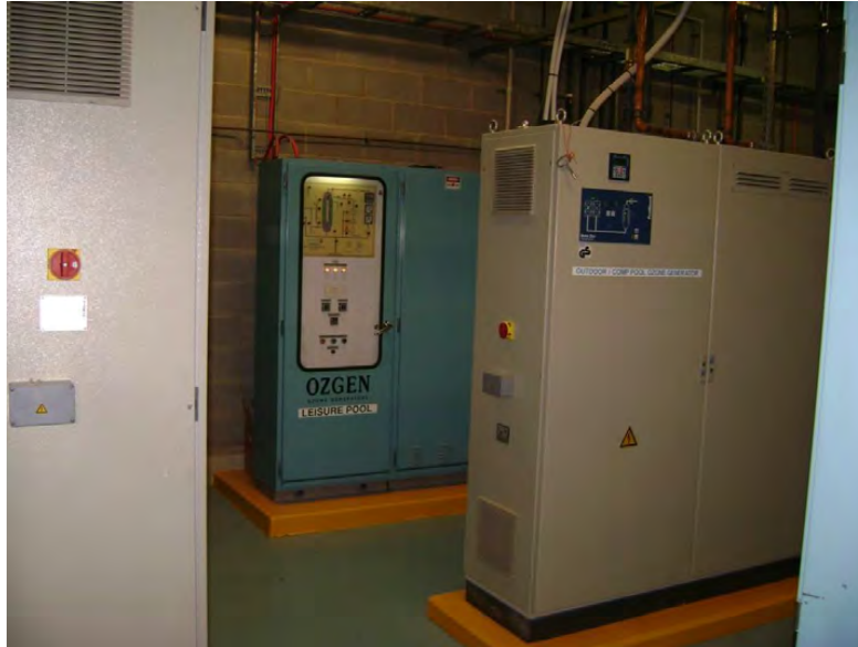
Typical ozone generator(s).
