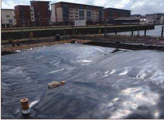
Gas membrane showing air/gas mixture pressurised
